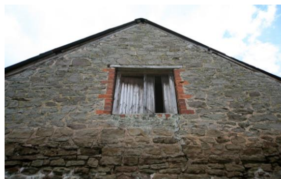
Fig.60 Typical rubblestone walling with red brick dressings as seen on an agricultural building on Chepstow Road
