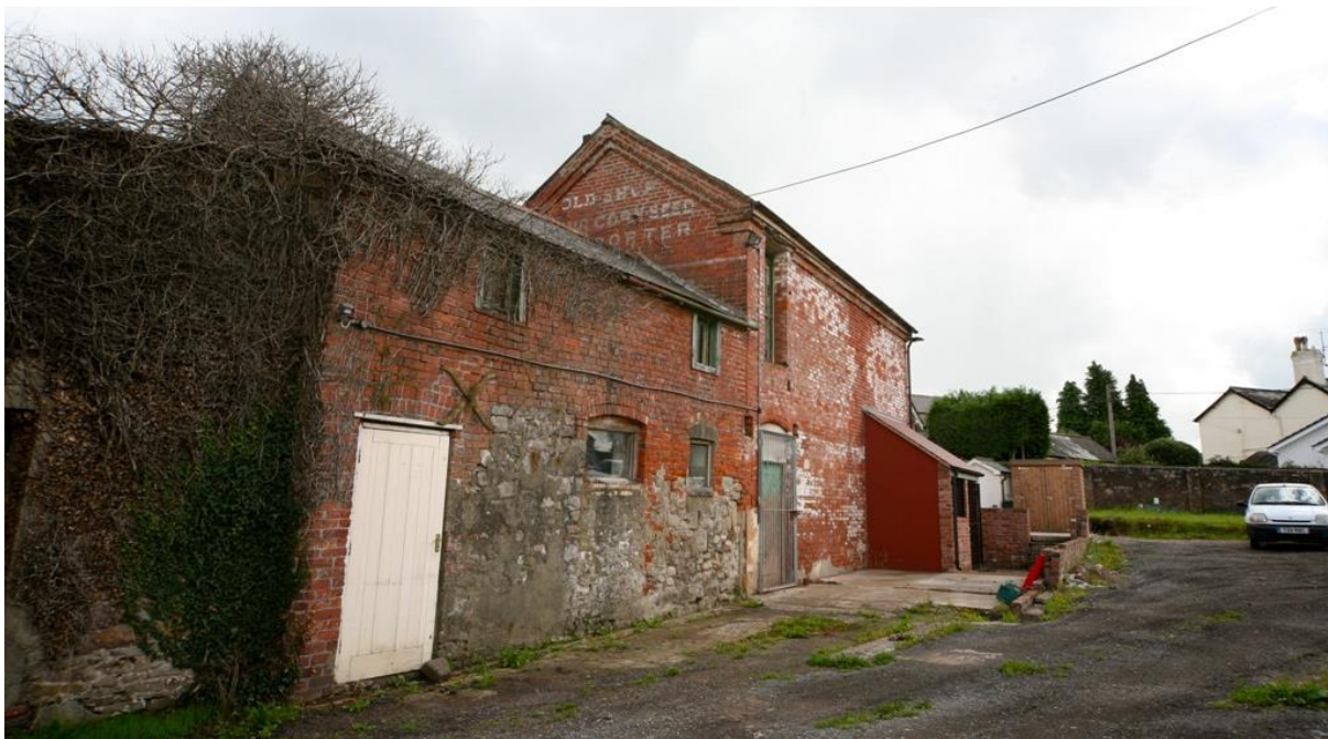
Fig.48 Attractive red brick outbuildings (listed) with historic painted signage are elements of significant local note
