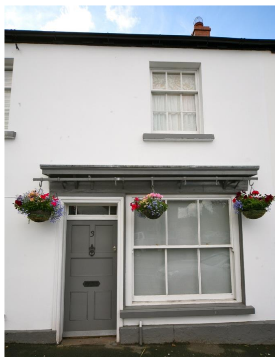
Fig.61 No.3 High Street: Good survival of traditional timber sliding sashes in the conservation area
